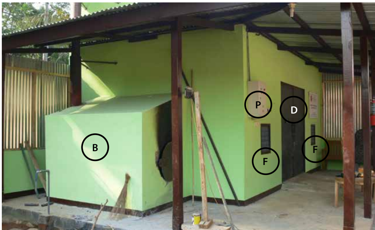
Notes: B=burner, D=door to chamber, P=power panel, F=fan
