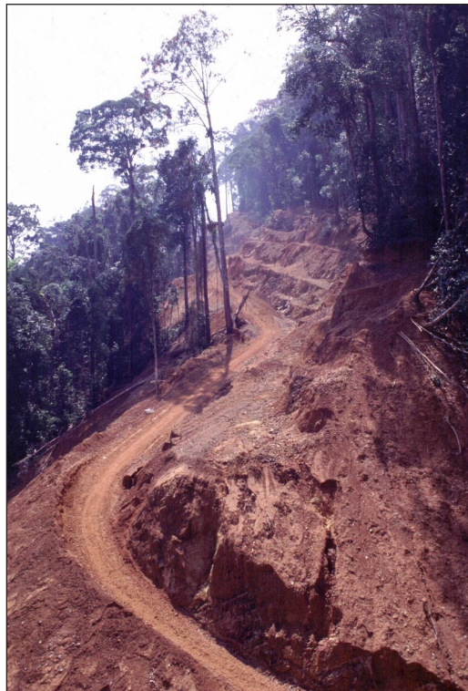
Photo 4: Excessive steep road grade
