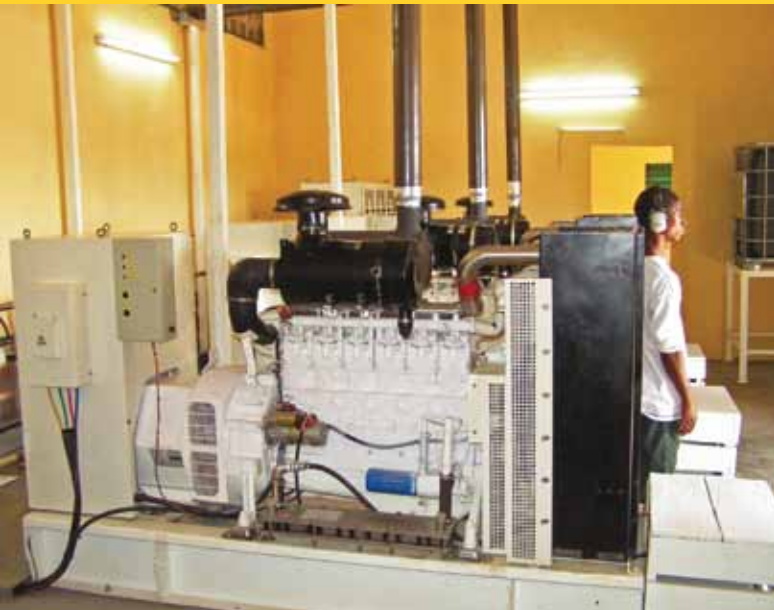
An operator stands in front of a bank of 100KW diesel generators designed to run on either diesel or jatropha oil at the Mali Folkecenter in Garalo, Mali. (Photo by Graham von Maltitz)
