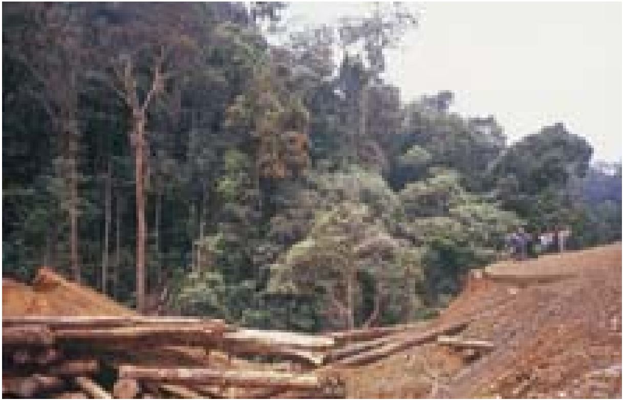
Poorly planned road construction
