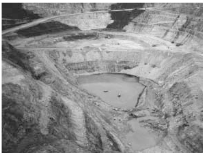
Plate 1. The Open Cut Mine at PT KEM. Photo taken by Anne Casson
