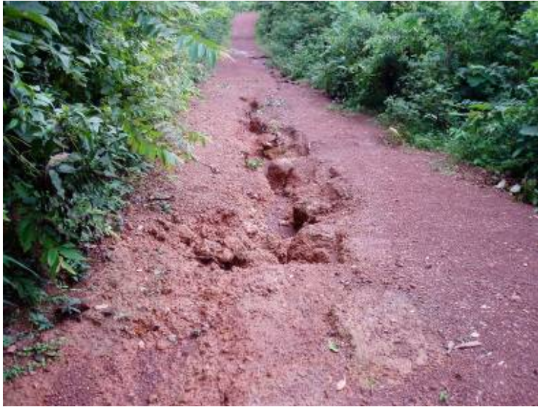
Plate 88: Significant patterns of gully erosion in sloping LPFL plantation access roads. Ban Pak Veng.
