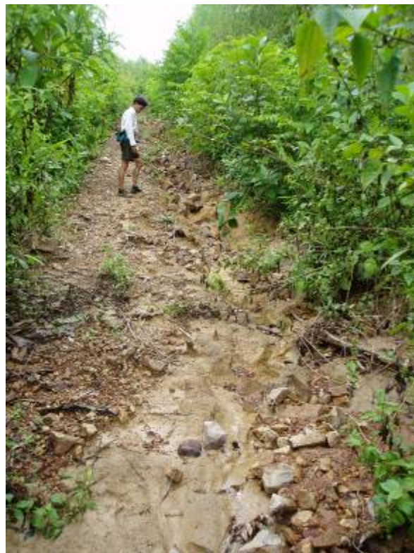
Plate 89: Gully erosion in year old Ban Pak Veng eucalypt plantations
