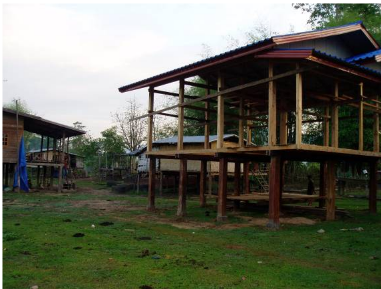
Plate 94: A new house under construction, built in significant part through the cash remittances from female wage labour in Thailand. Ban Pak Veng.
