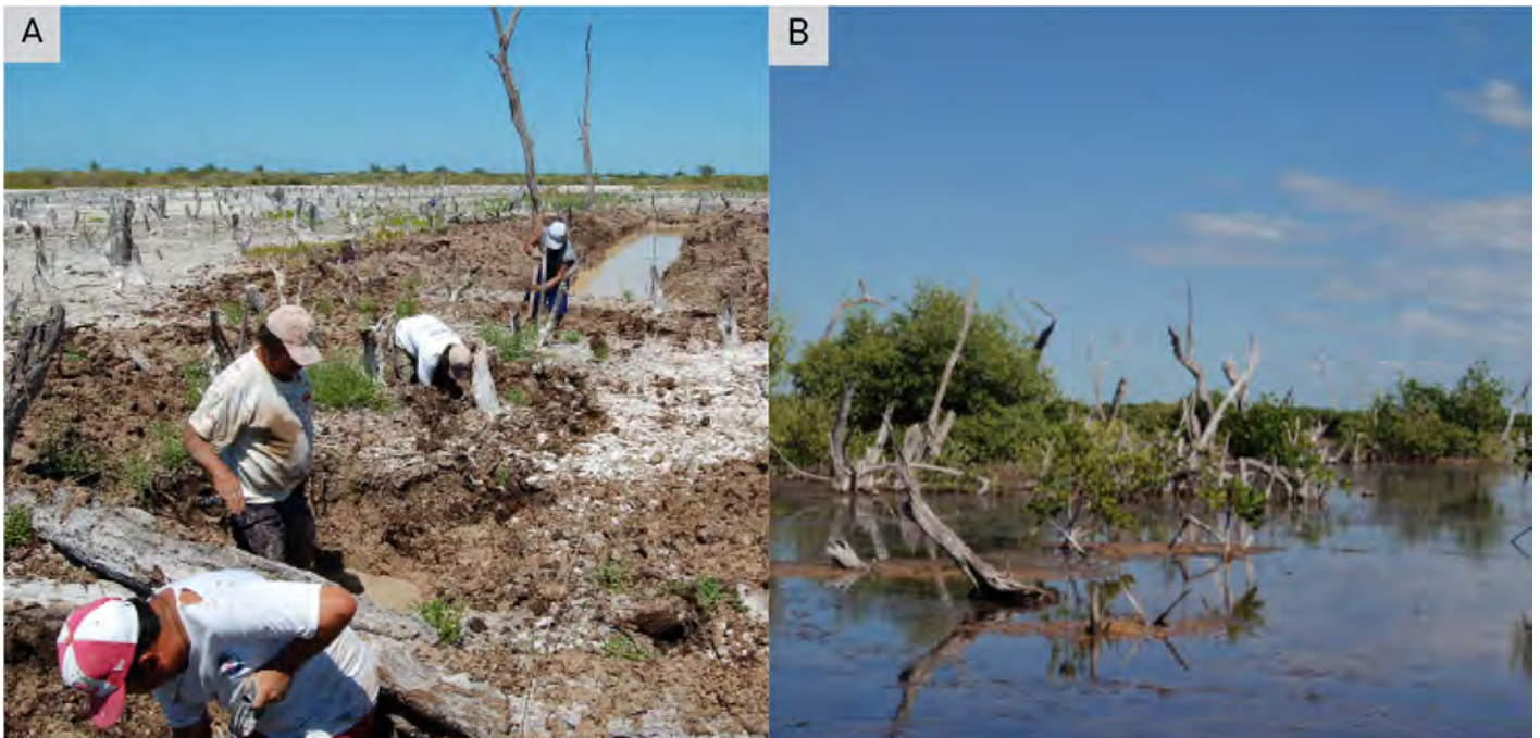
A) Construction of the main channel; B) main channel one year after the restoration actions started.
