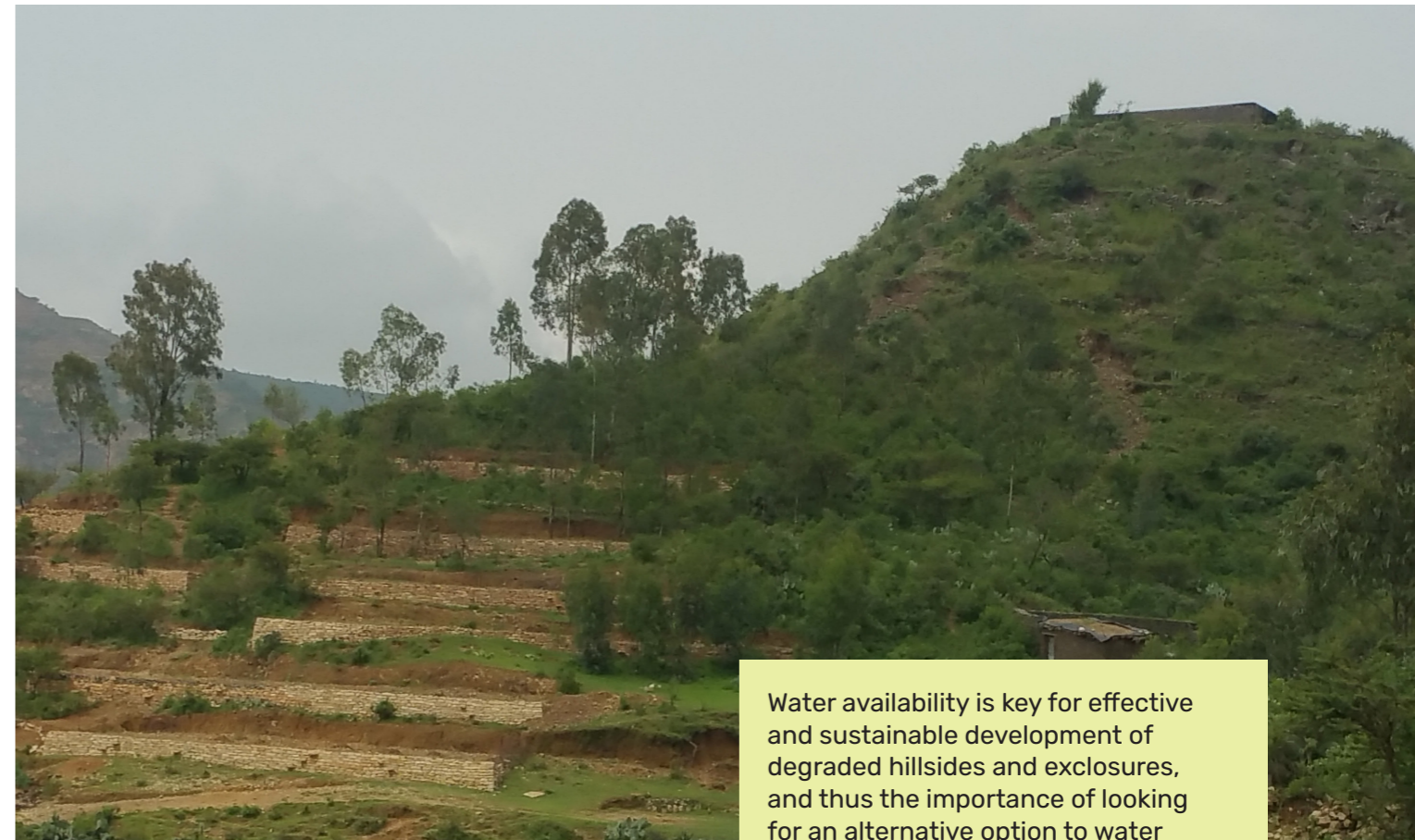
Partial view of piloted low-cost and innovative rainwater harvesting reservoirs at the top of a mountainous hillside to irrigate high-value trees and grasses during the dry season. The reservoir has a capacity of 72 m 3 or 72,000 litres. Whenever there is a small flat space at the top of a given mountainous hillside/exclosure, it is possible to dig a reservoir, build a corrugated iron roof shelter, and direct rainwater to the reservoir.
