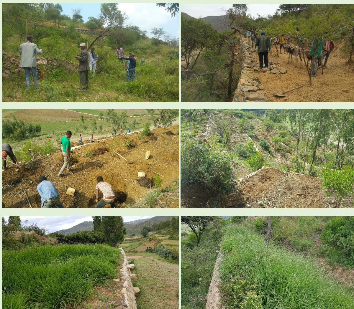
Figure 6: Partial view of hillsides and exclosures; experts and community representatives discuss the design of bench terraces to be constructed and, community engagement during the construction (upper), planting of high-value biomass-producing and nutritious fodder grasses and management of existing vegetation within and between bench terraces (middle) and growth performance of planted fodder grasses (lower).
