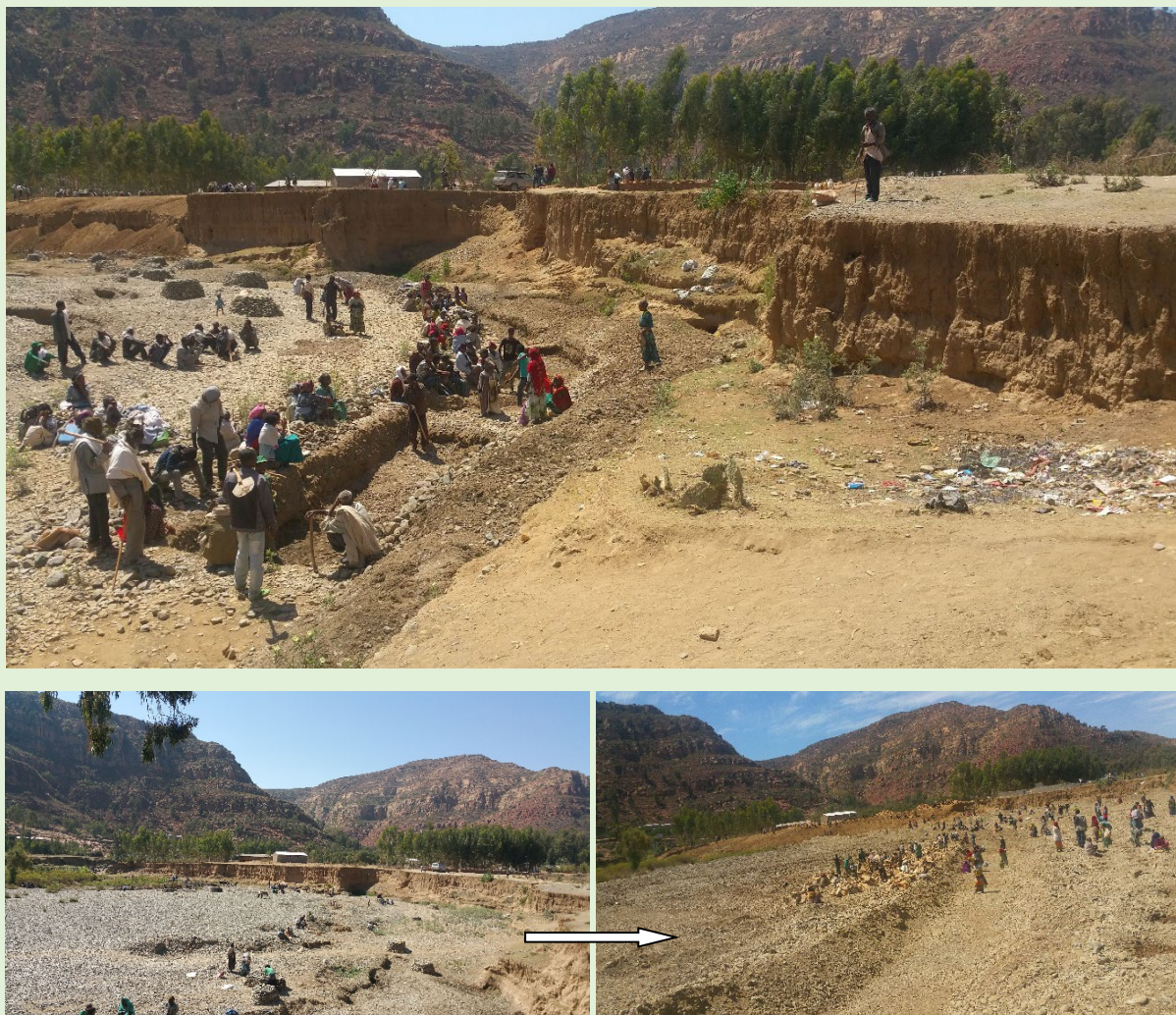
Figure 3: Partial view of active participation of communities in the reclamation process of wide and deep gullies along the Gergera watershed
