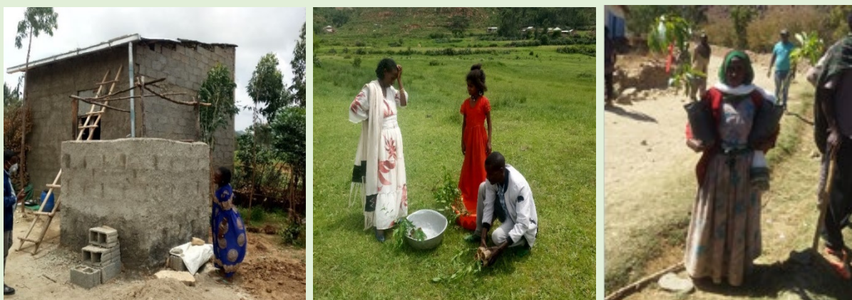
Figure 12: Partial view of roof water harvesting structure constructed by women-headed households (left) to promote home garden agroforestry. Women receiving high-value, quality fruit seedlings to plant in their homesteads (middle and right)
